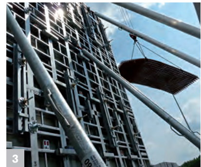
3 Quick pouring without restrictions due to a load capacity of 100 kN/m 2 throughout the system
